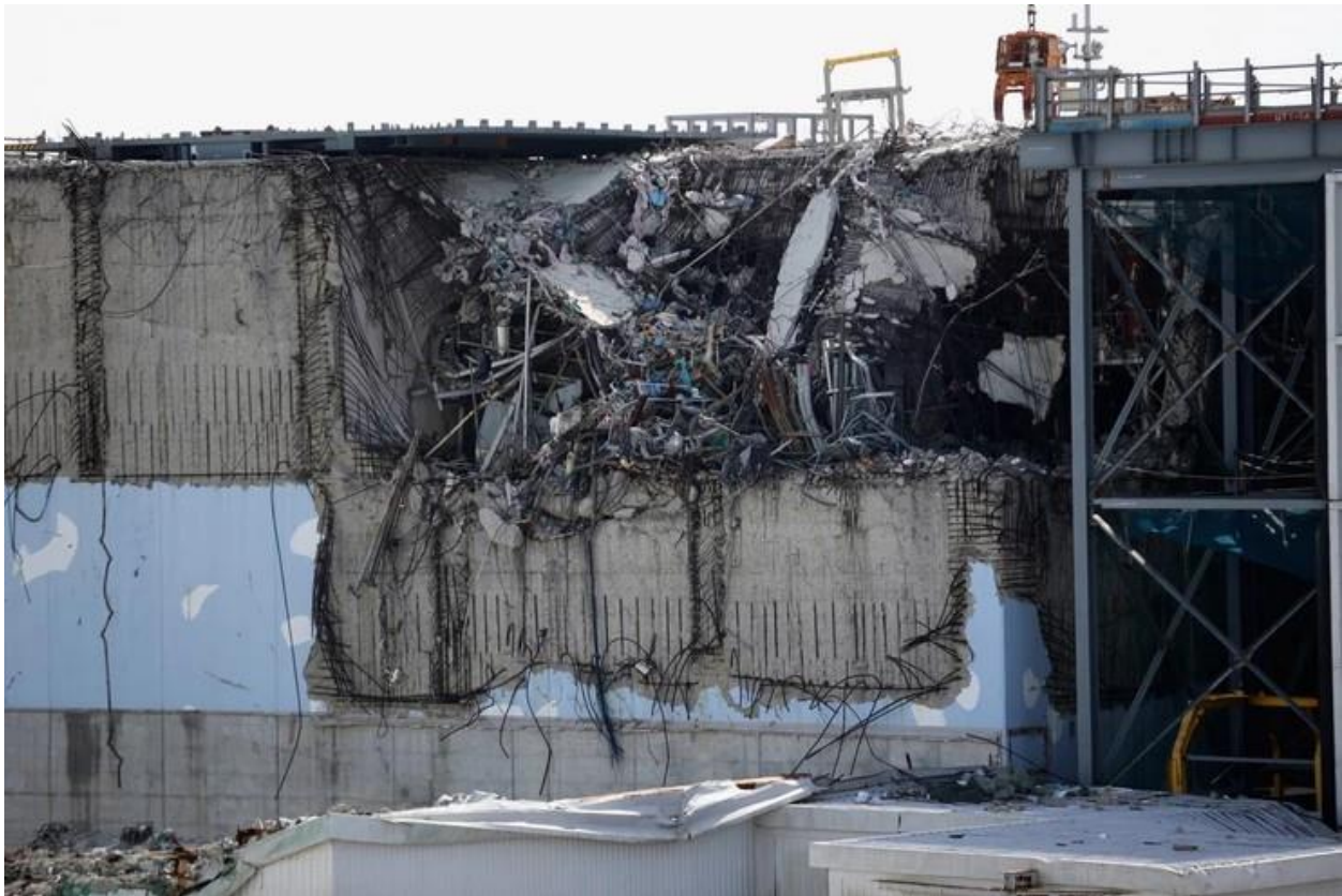
Damage to No. 3 reactor building at Fukushima Daiichi nuclear power plant, March 2011
