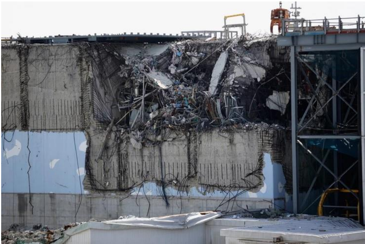
Damage to No. 3 reactor building at Fukushima Daiichi nuclear power plant, March 2011
